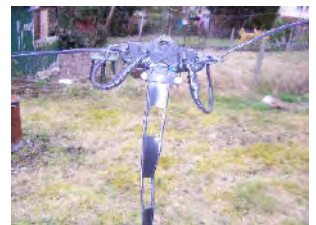
At the top of the feeder, after weather-proofing - not pretty but waterproof!!
